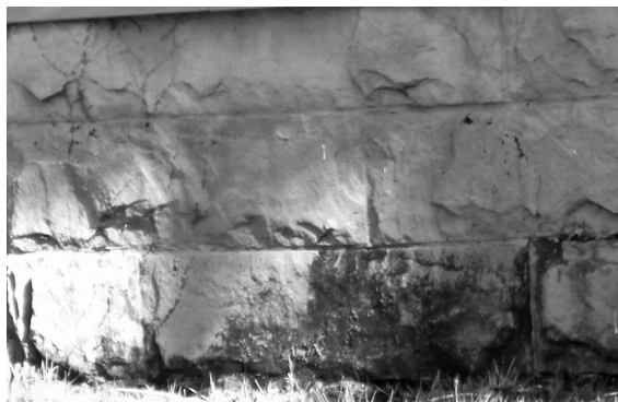
Figure xvi: The natural stone foundation at 2320 Bellfield Ave. supports its 19th century build date (Peskin, L.)
