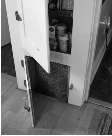
Figure viii: The in-wall sweep chute at 2930 E. Derbyshire Road, a Ray Hummer built double, displays two themes of this story: preservation of original features in Heights doubles and their high comfort and convenience level. (L. Peskin)
